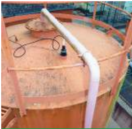
dB Transducer mounted onto an oil tank at Leigh Infirmary
